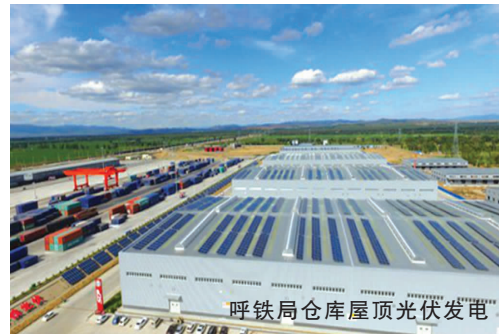
“呼铁局仓库屋顶光伏发电”
